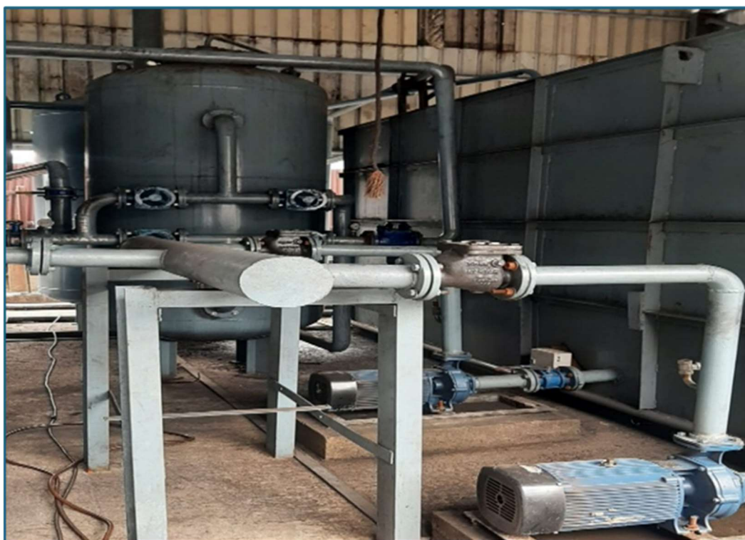
Fig. ZLD system in use
