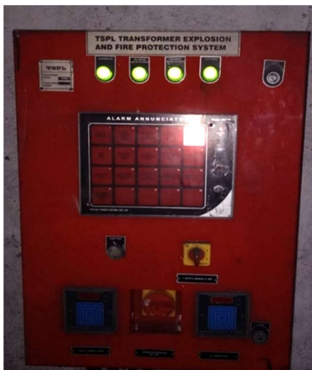
Fig. Transformer Explosion and Fire Control System
