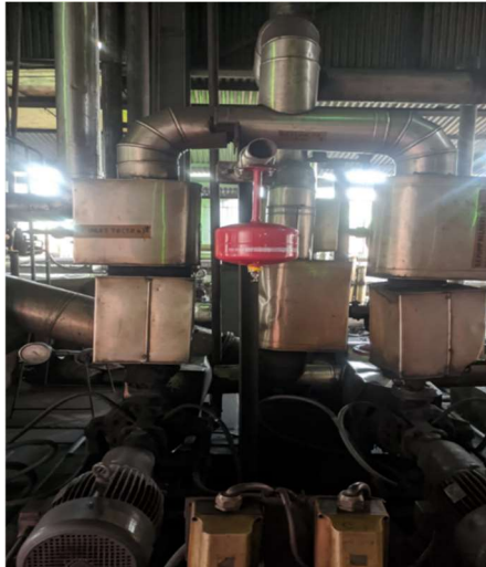
Fig. Automated Fire Suppression System
